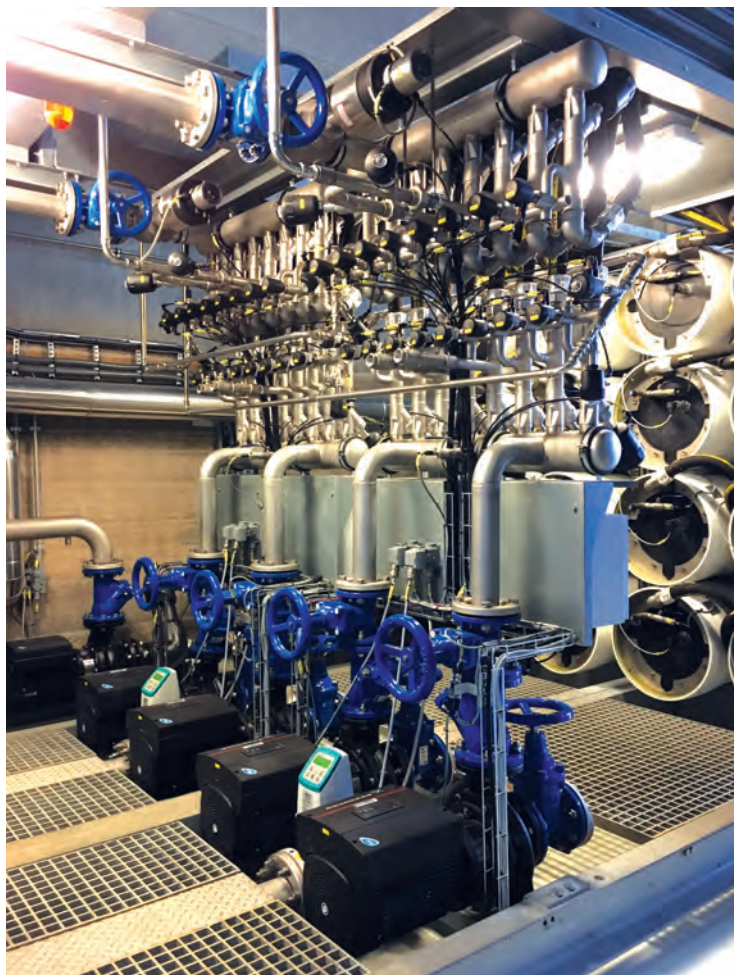
Industrial pumps, like the Grundfos Biobooster above, play major roles in various F&B operations.
